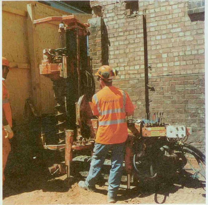
A mini pile installation technique was found to be the quickest and cheapest solution for both the soil nailing and piling
