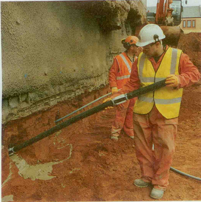
Drilling soil nails into the rock beneath the warehouse avoids the need for a retaining wall between the buildings
