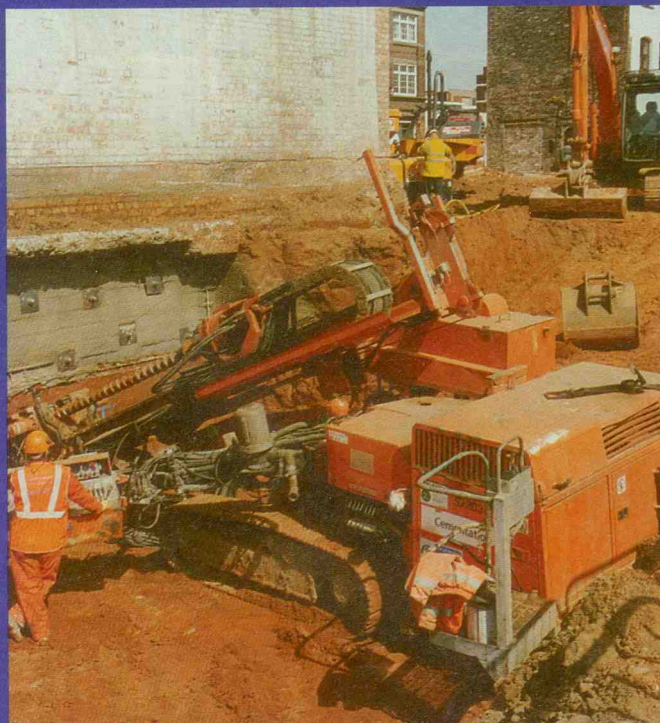
The first stage of the soil nailing technique involves rotary drilling a 3m long hole, declined at 20 degrees beneath the building. This 140mm diameter bore is immediately filled with a neat cement grout.
