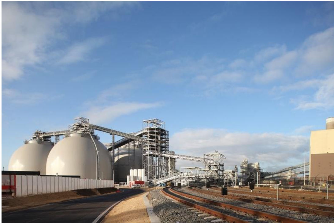
New train line around site to increase supply chain efficiency and accommodate the redesigned trains
