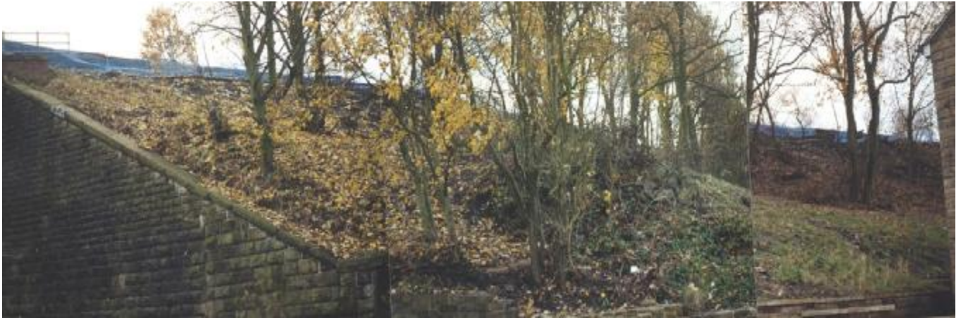
Figure (i) - Original Embankment Prior To Any Remedial Works (Late 1997)
