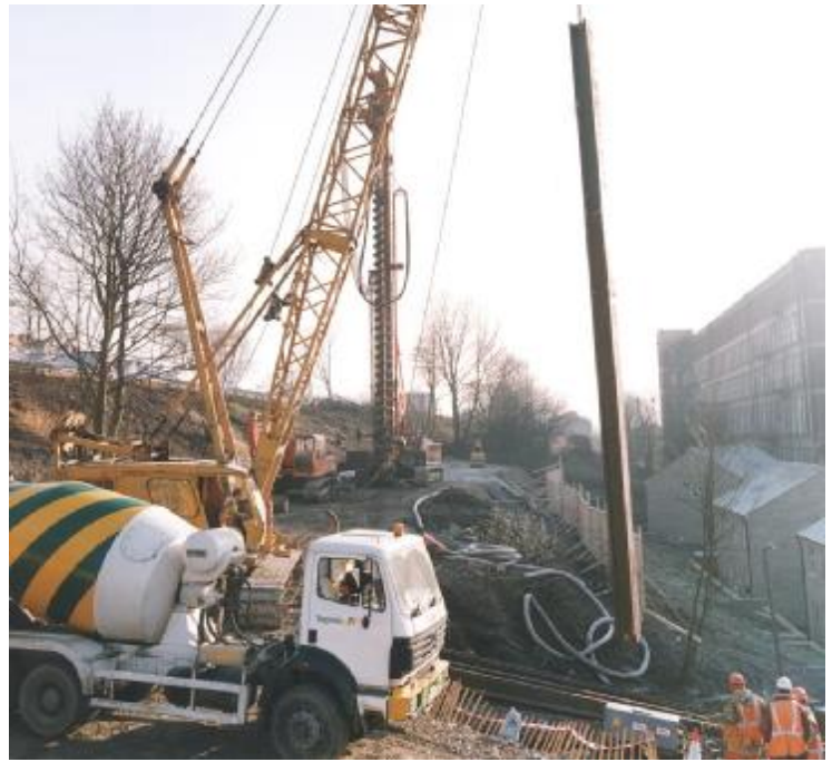
Figure (vi) - Lifting of Universal Column (note the steepness of the overall slope)
